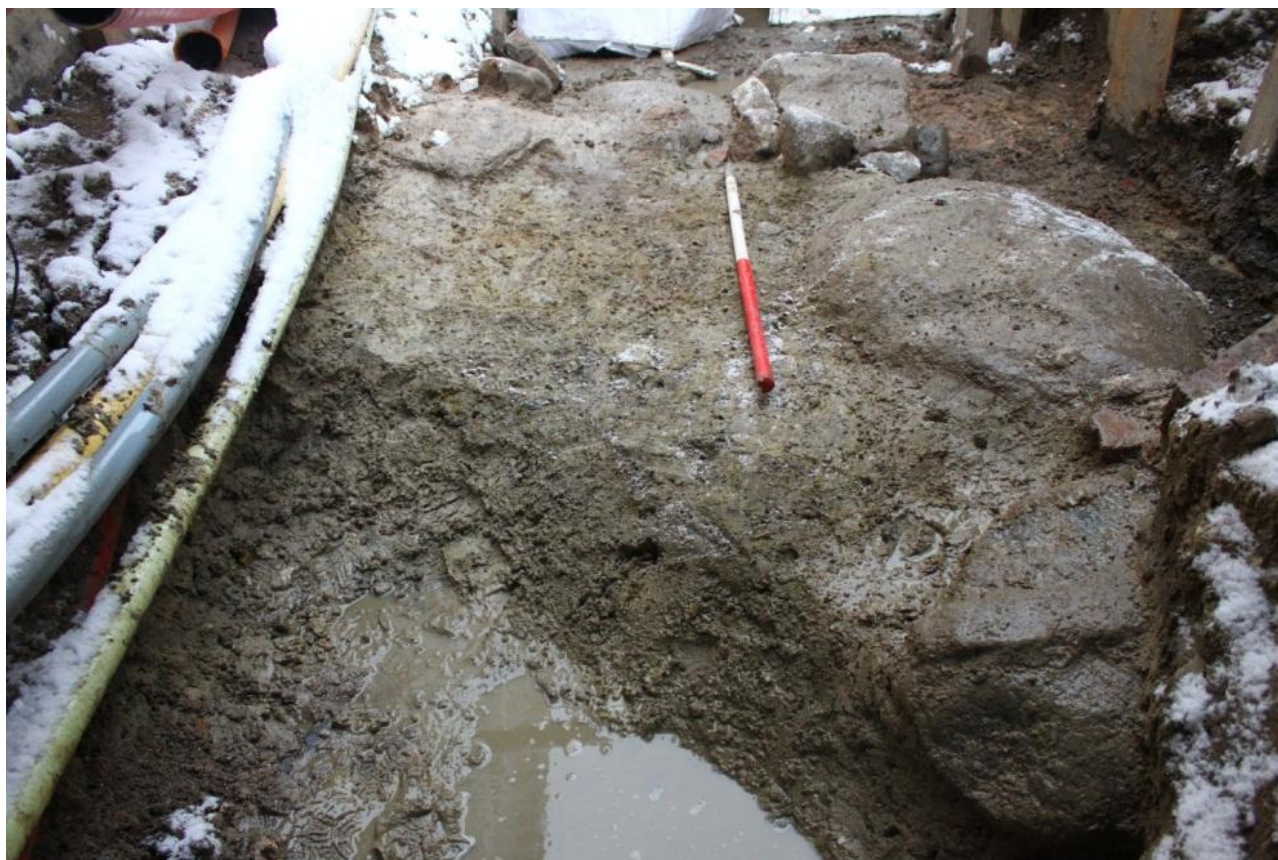
Fig. 278. Granite boulders in foundation (SS30007) in building G-235, facing north. Photo: Museum of Copenhagen.
