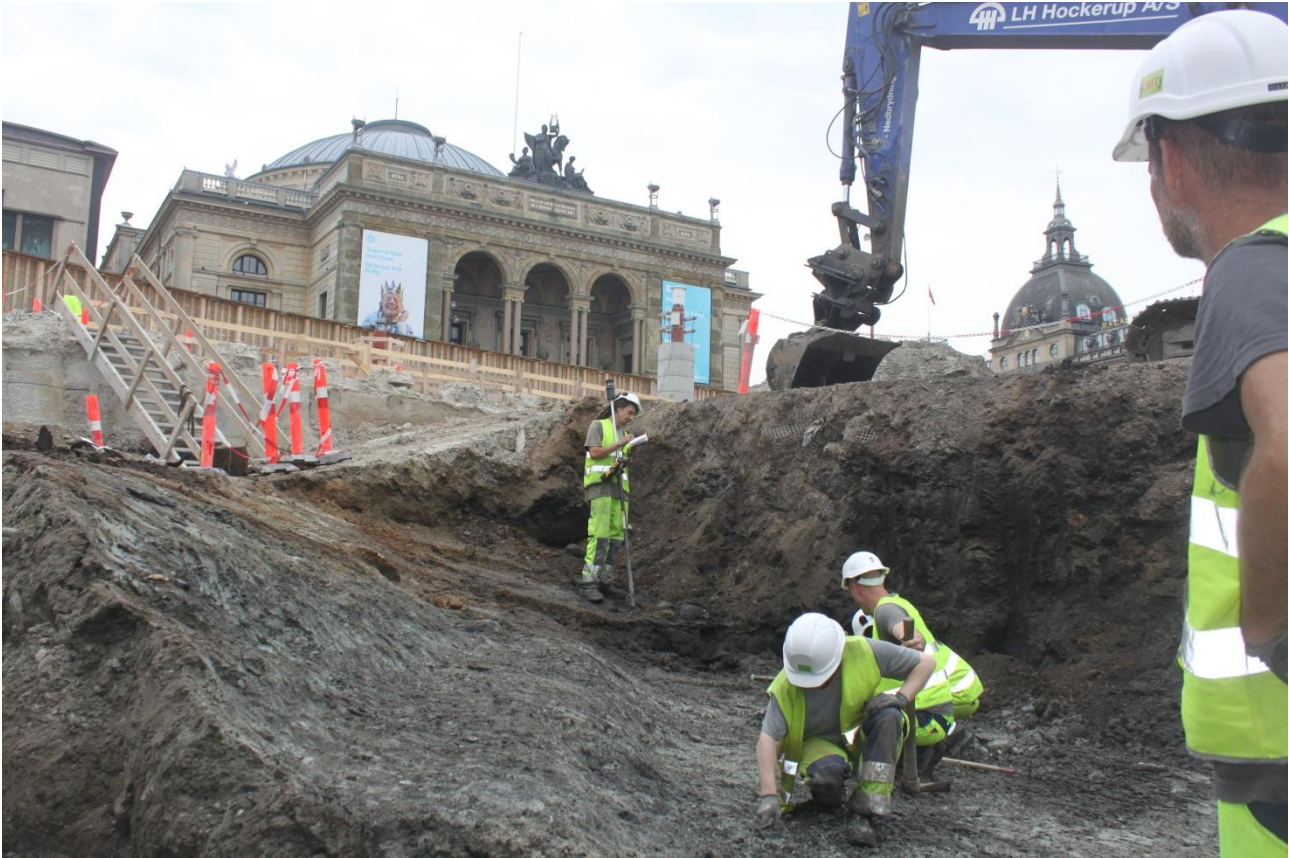
Fig. 221. Exposing and cleaning the eastern stepped side of the 17 th century moat, facing south with the Royal Theatre in the background. Photo: Museum of Copenhagen.
