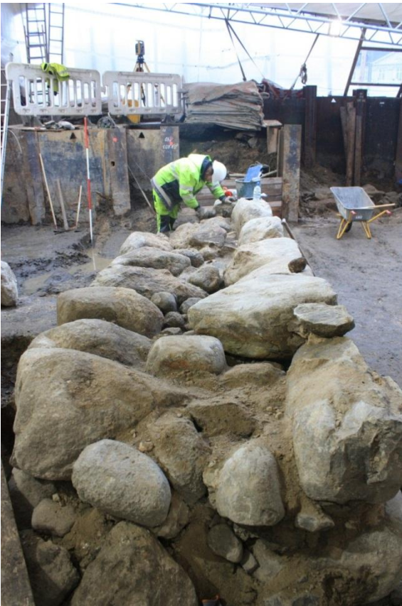
Fig. 104. Investigating the double faced wall in the northern part of the building with infill of mortar and stones, facing east. Photo: Museum of Copenhagen.
