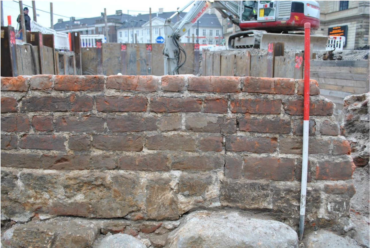
Fig. 89. Detail of brick wall and limestone coursing, facing east. Photo: Museum of Copenhagen.
