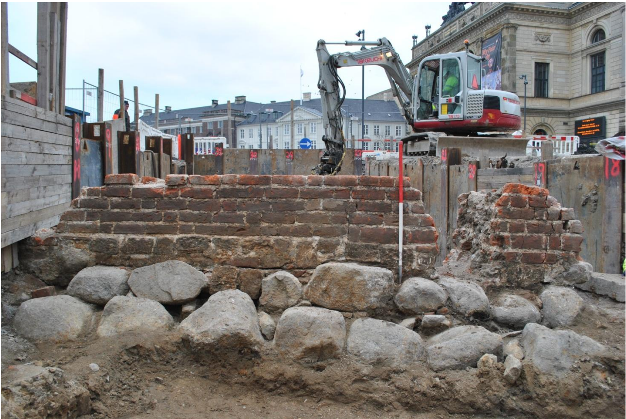
Fig. 84. General view of brick wall and foundation, facing east. Photo: Museum of Copenhagen.
