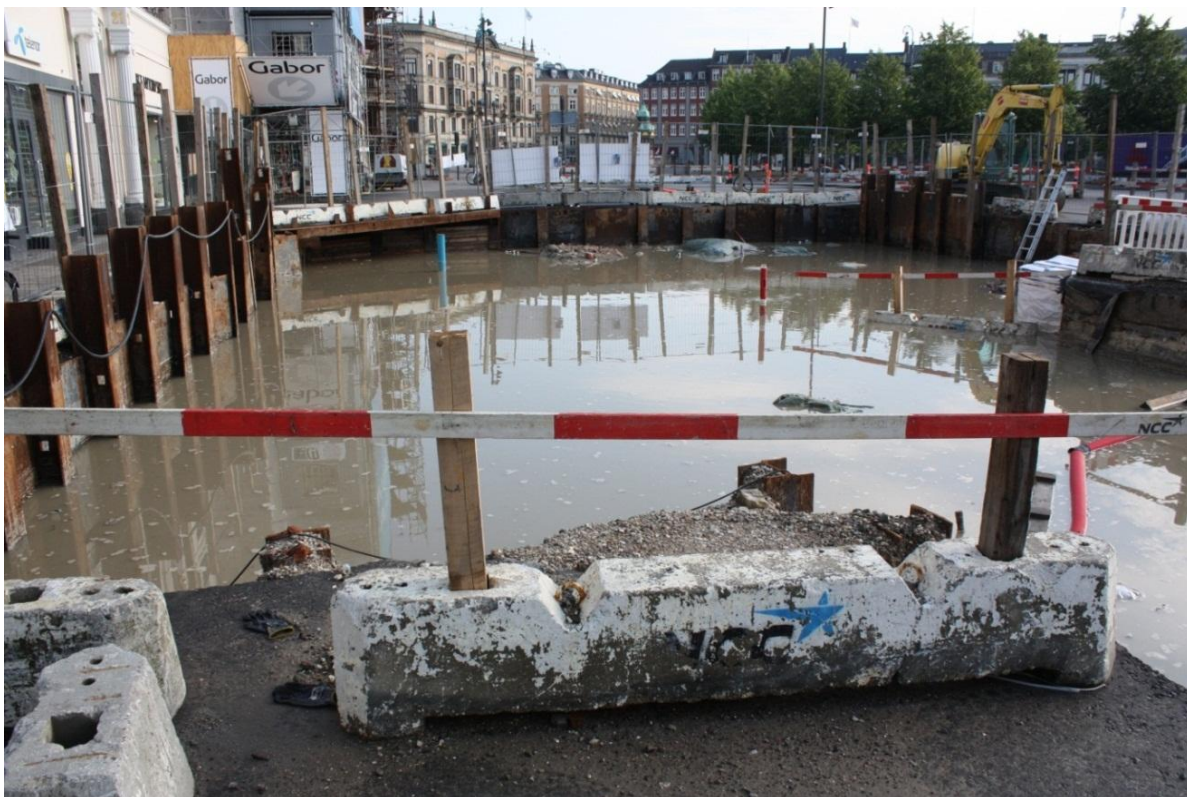
Fig. 23. A Field Leader's nightmare. Subarea phase 45B after the flooding 2 nd July 2011. Photo: Museum of Copenhagen.
