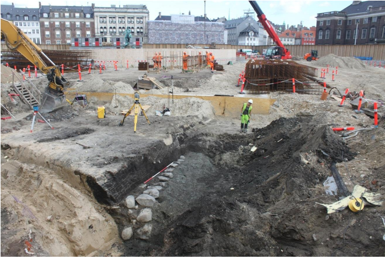
Fig. 25. Overview Guide Wall trench with part of the bastion and 17 th century moat, facing NE. In the left handside corner – modern sand in a central heating trench. Photo: Museum of Copenhagen.
