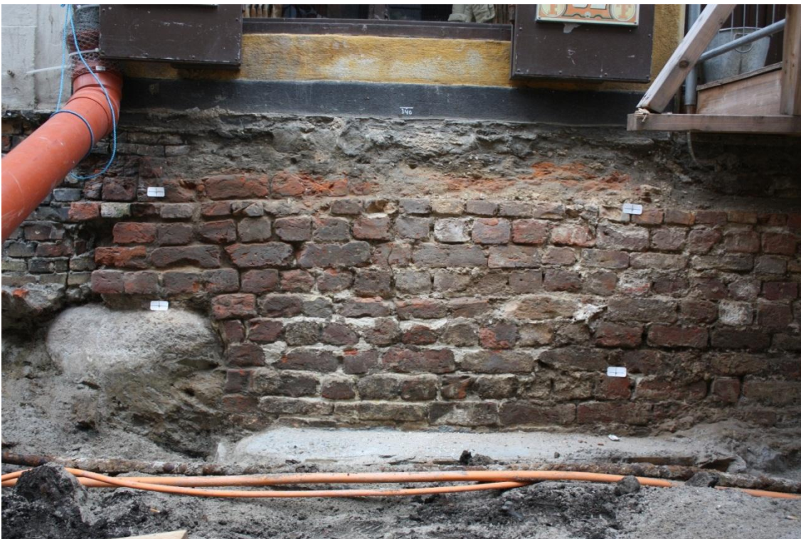
Fig. 329. Exposed brick wall and foundation stone at Hviids Vinstue, facing north. Photo: Museum of Copenhagen.
