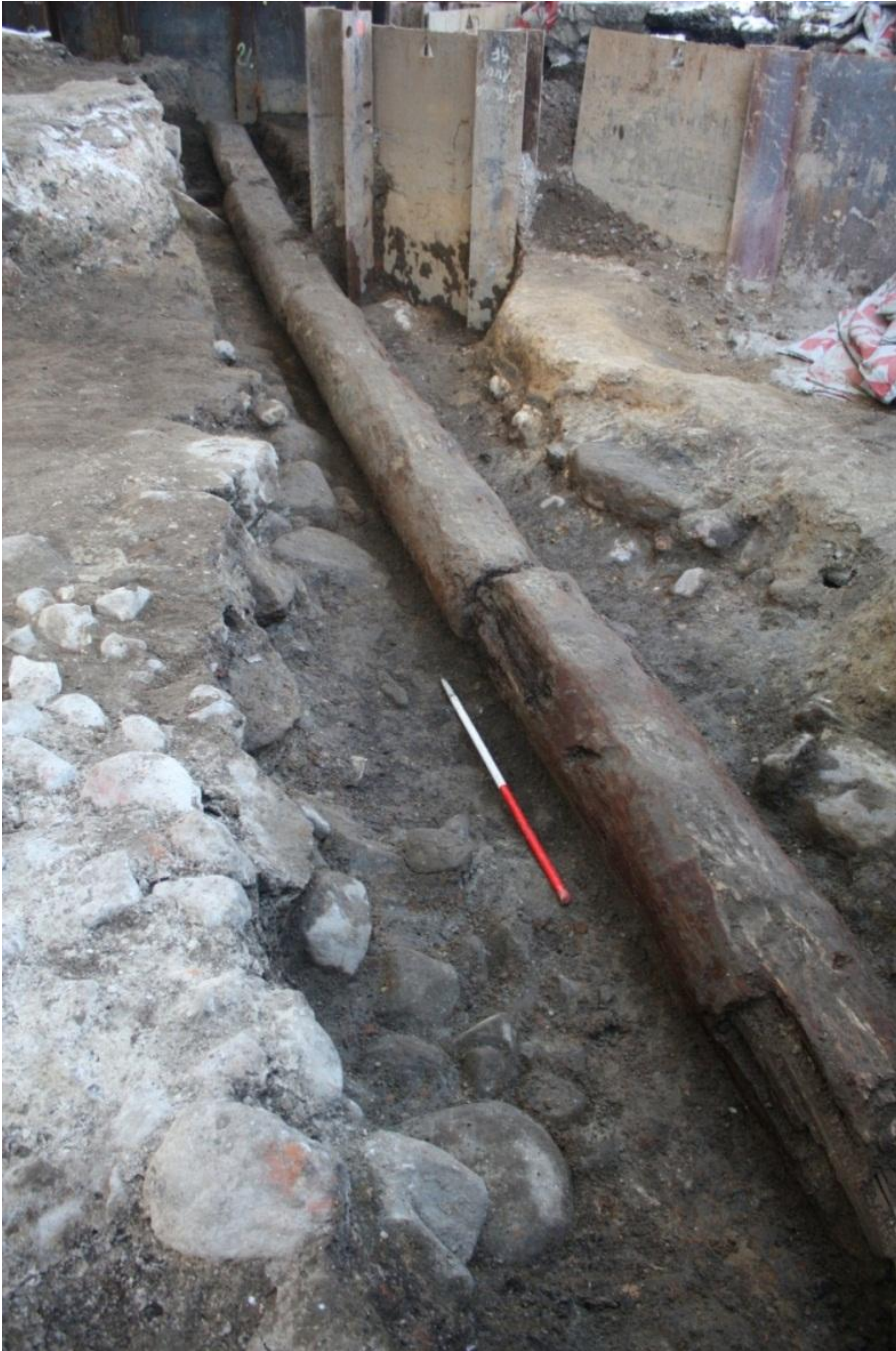
Fig. 349. One of the main pipelines at Kongens Nytorv. Wooden water pipe (ST30444; SG-336) with construction cut through the foundations of 17 th century Østerport, facing SW. Photo: Museum of Copenhagen.
