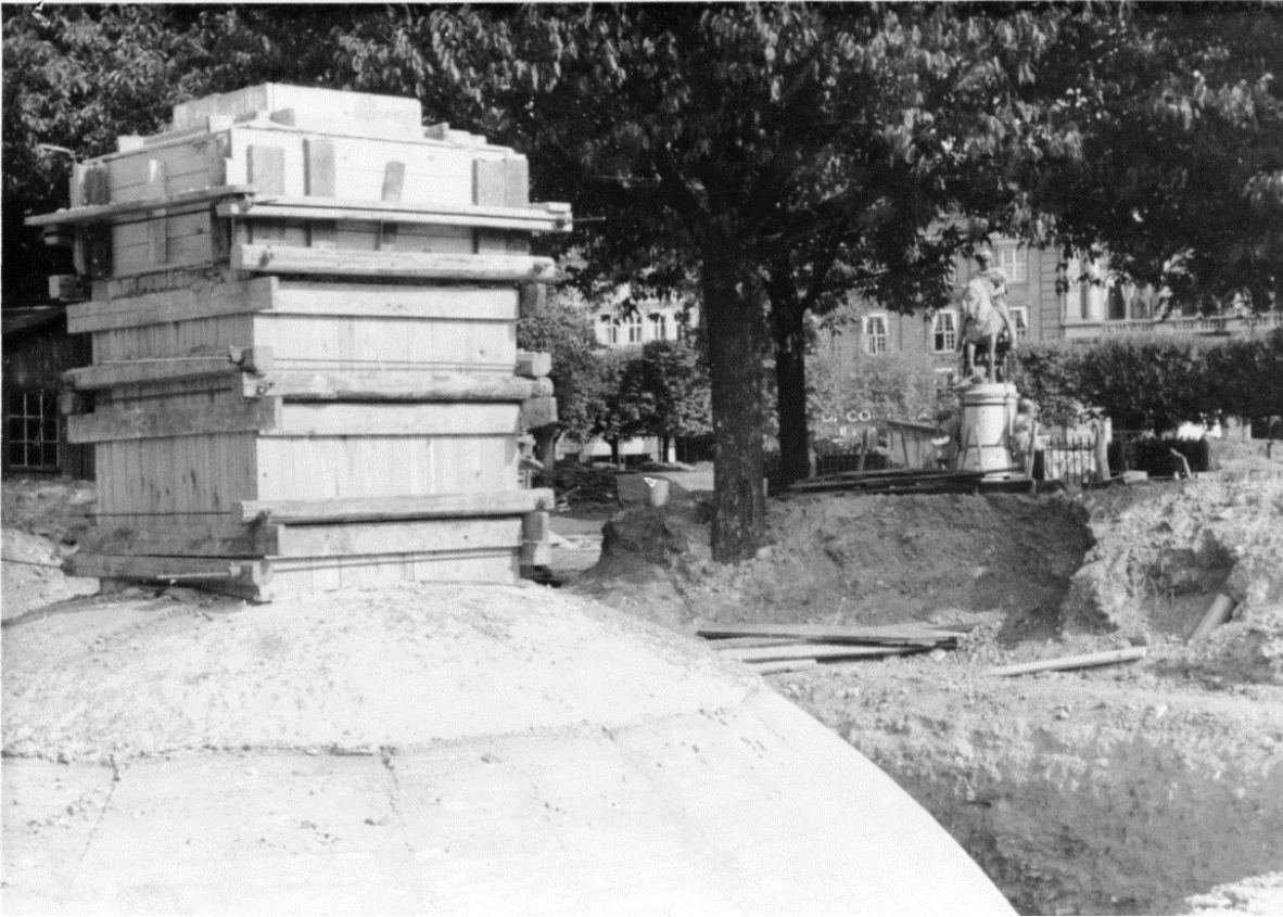
Fig. 351. Dome shelters under construction at Kongens Nytorv in 1944. From Museum of Copenhagen.
