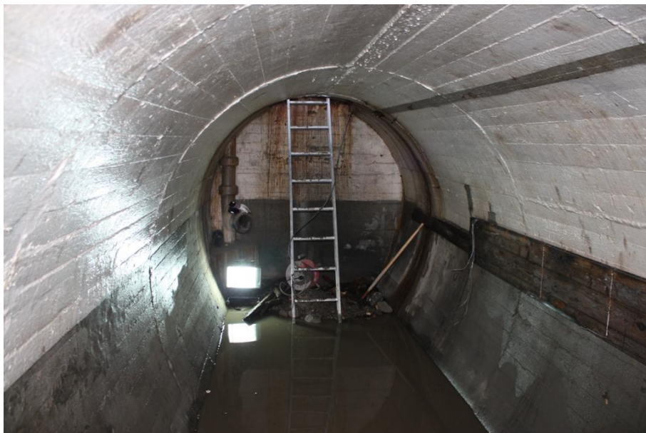
Figure 167 The northern end of shelter Group 43. Note the wooden panel and wires to the right, and the ceramic pipe in the corner.
