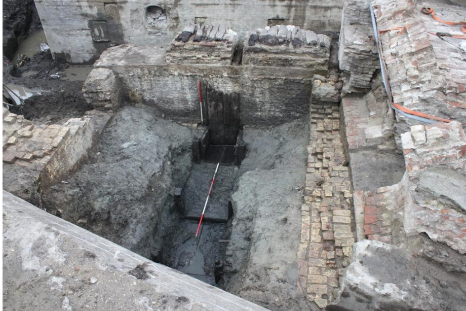
Figure 127 The lower sluice element of the head race exposed within the bridge arch. Seen from NW
