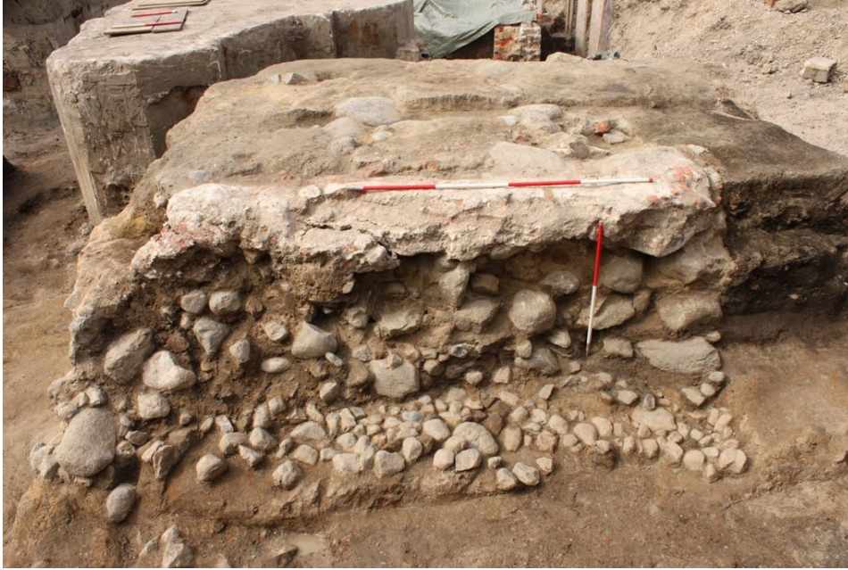
Figure 84 The outer foundation of gate Group 111 as it survived, truncated both lengthways (by wooden waterpipe) and to the southeast (left in photo)
