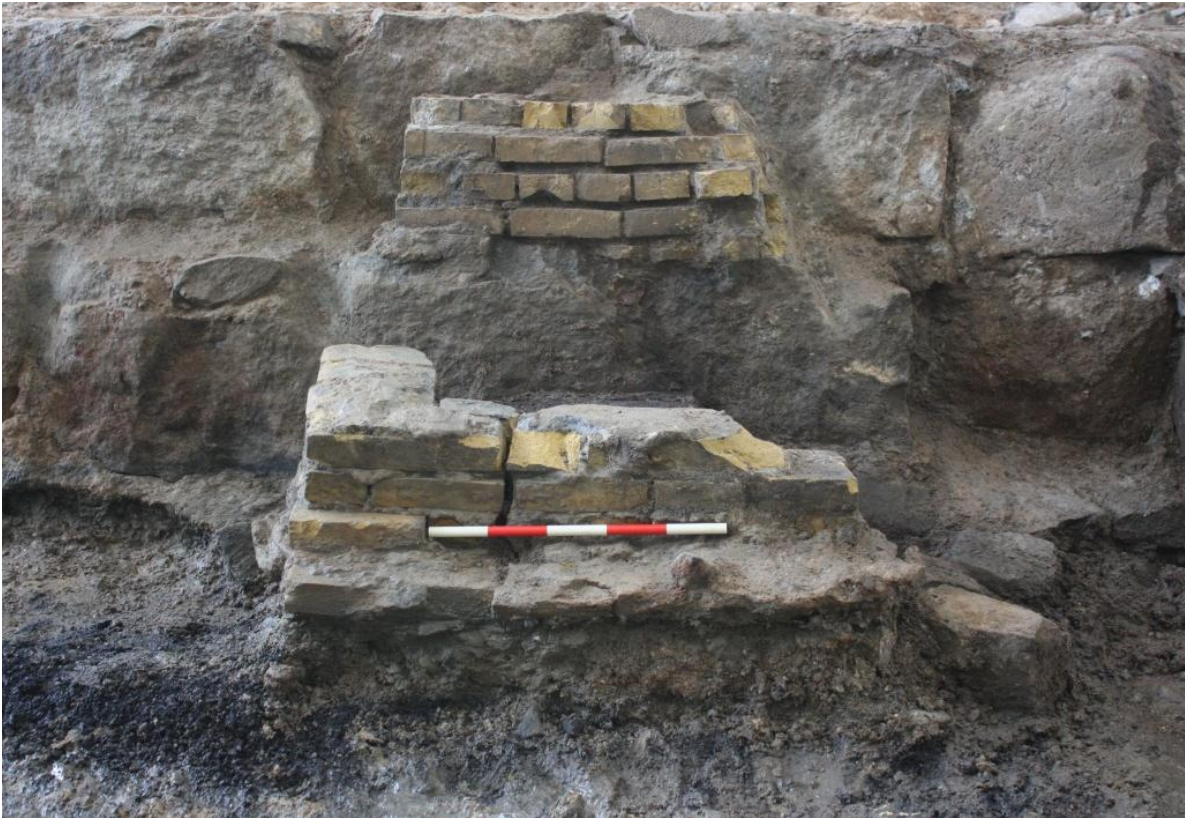
Fig. 148 Brick street light foundation G625 abutting and built into the earlier 1880s stone harbour wall, looking south. C03_20140204_7913 (cropped)
