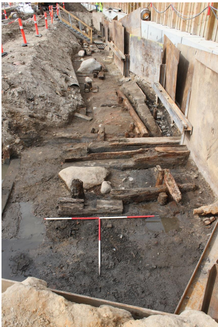
Fig. 375 Excavation of the Guide Wall trench, September 2012. Trenches 2B and 3. Looking SW. C19_20120824_3707
