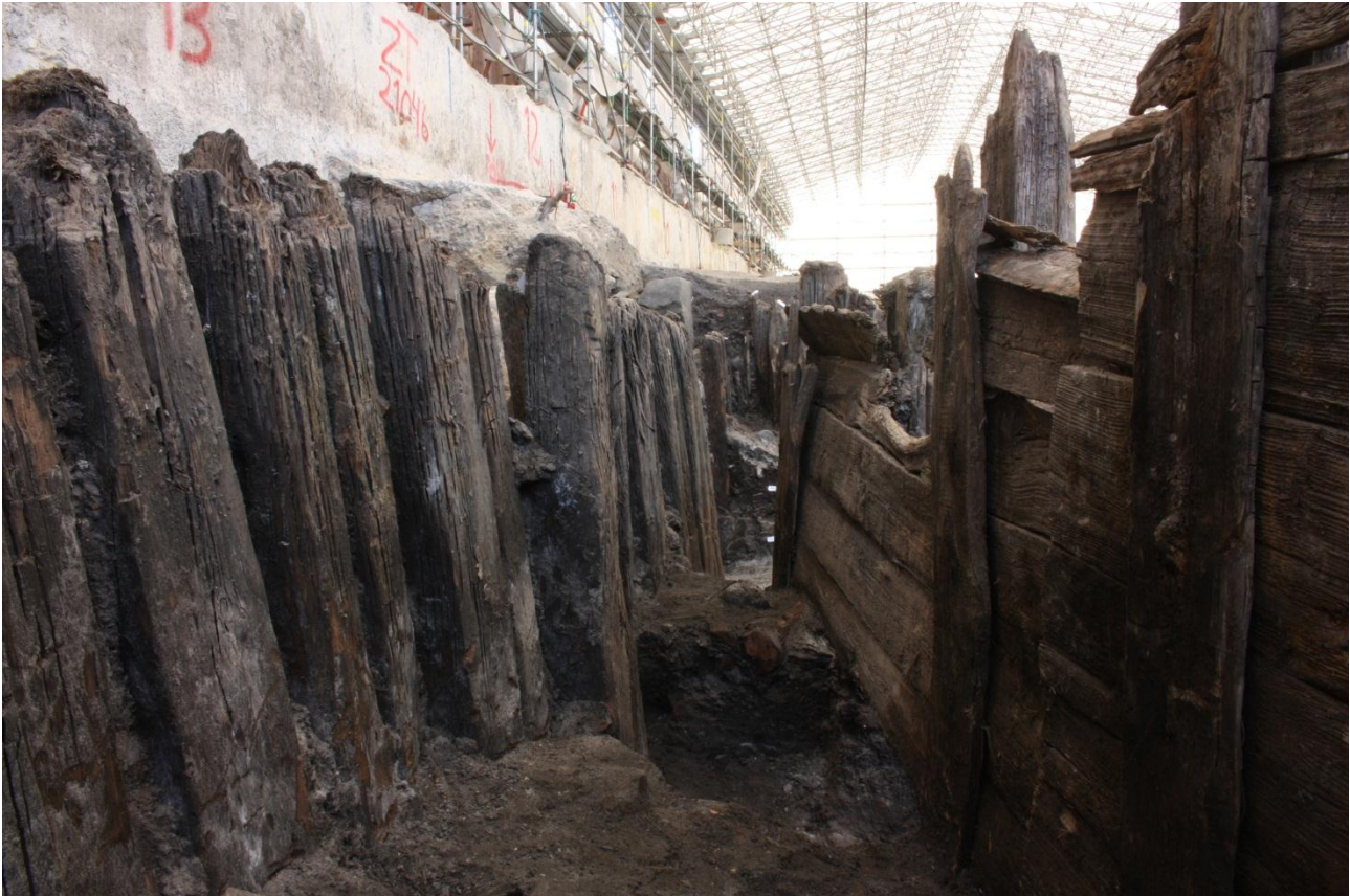
Fig. 61 Working photo of the excavation between G602 and G674 looking NE. Note the majority of the backfill has been removed. C03_20140624_11196.
