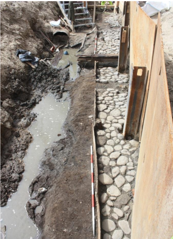
Fig. 54 Working photo of Road Group 430 looking SW in Trench 1 of the Guide Wall trench. The photo comprises road deposit 11789 at rear and road deposit 10493 in foreground. C03_20120723_5083
