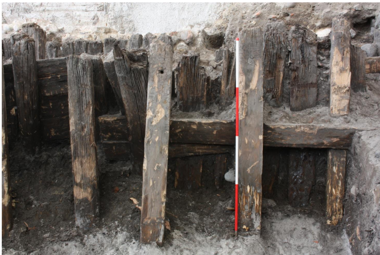
Fig. 64 Close up of harbour bulwark G648 next to the baulk. The photo is centered on an area of repair shown by horizontal plank ST41884 and three vertically set planks (ST39435, ST39413, ST55582) used as the plank's support. The photo is looking N. C03_20140613_10920
