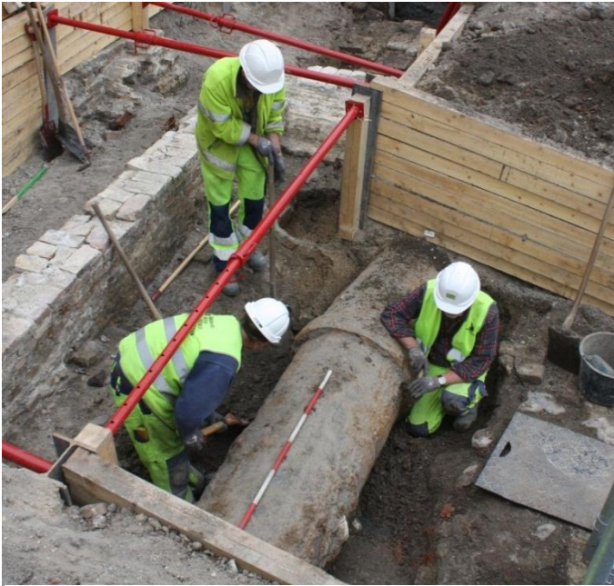
Fig. 363 Working shot showing the gas pipe cut SC9090, G720, in the Guide Wall trench as it was found during excavation, viewed from the southwest. C03_280612_4589 (cropped)
