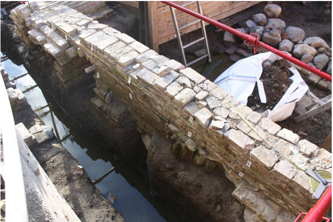
Fig. 258 A working photo showing the recording of wall SG420 with overlying rebuild SG418, viewed from the northwest. The two culverts SG223 and SG423 can be seen in the top left of the photograph. Looking SE. C03__20120718_4967
