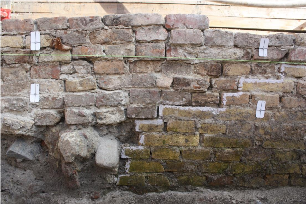
Fig. 268 The rebuild SG418 over wall SG420: the deconstruction of SG420 on the diagonal can clearly be seen, viewed from the south. The poorer quality of the overlying brickwork is evident when contrasted against the earlier wall. C03_20120717_4941
