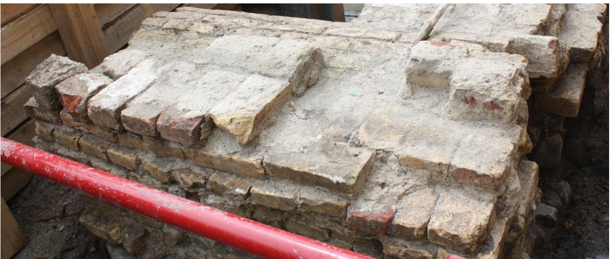
Fig. 266 SS12104 of SG409 along the east side of culvert SG423. Looking SW. The red bricks in the upper courses of the wall are clearly seen. C03_280612_4658 (cropped)
