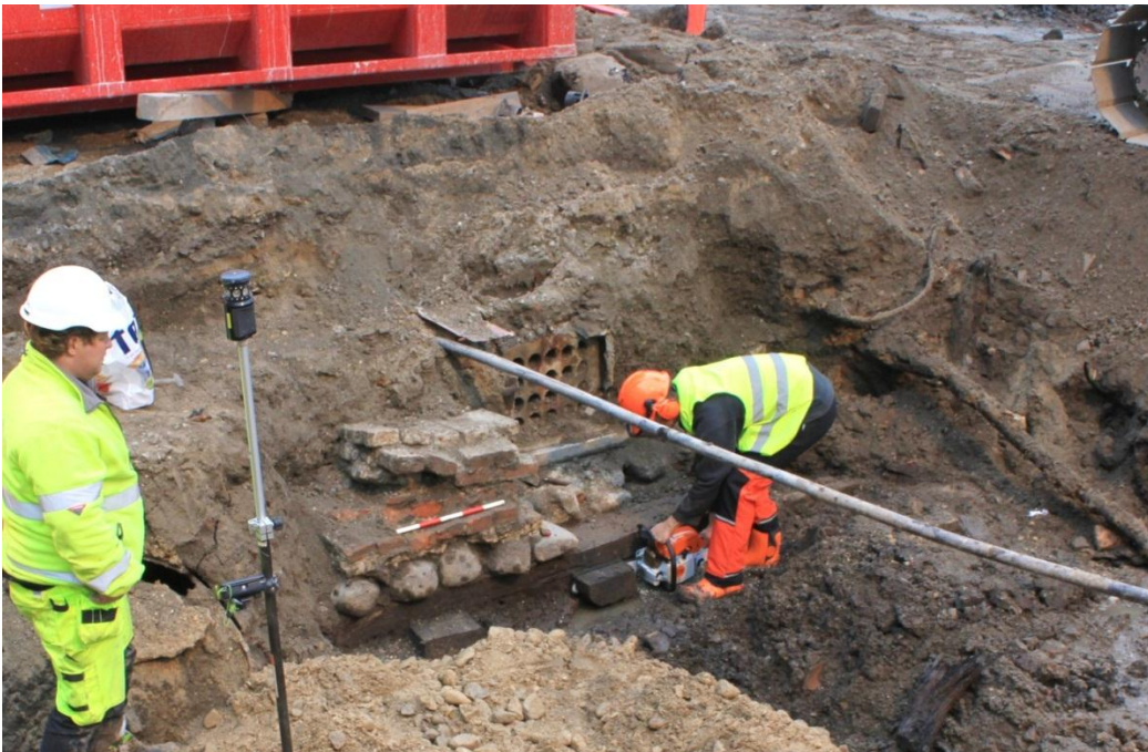
Fig. 7 Working photo of the Oil Container trench and the sawing of wood for a dendrochronological sample. C19-20121123_4354.
