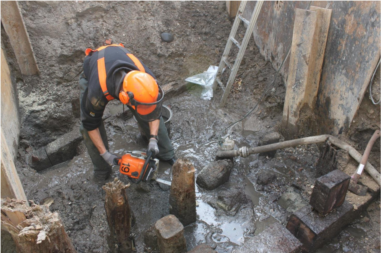
Fig. 182 Photo displaying the use of chainsaw cutting the timbers for analysis. Guide Wall excavation 2012. C19_20121018_4271
