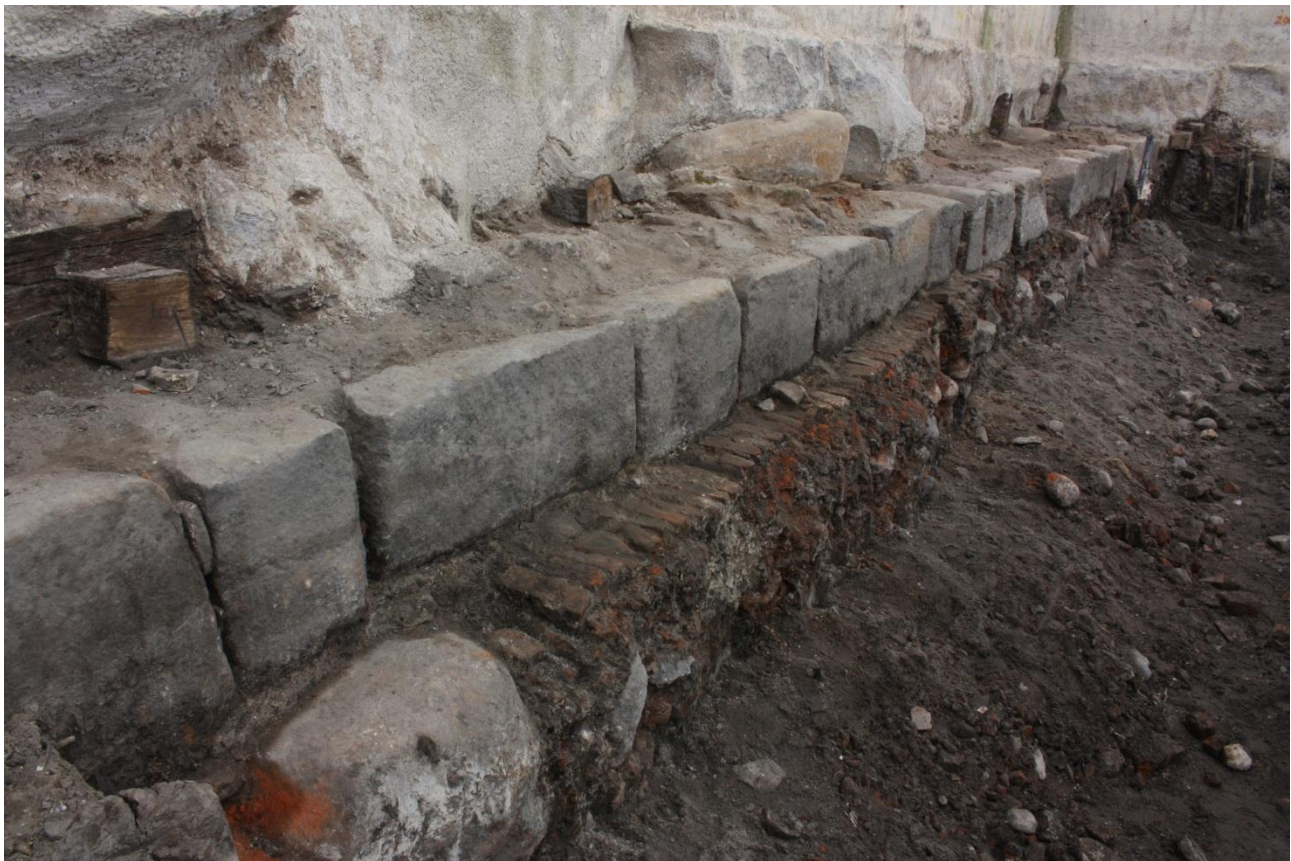
Fig. 72 Photo of eastern end of wall G532 after bulwark G602 was removed Photo shows the different construction methodology to areas in the centre and west. C03_20140613_10888
