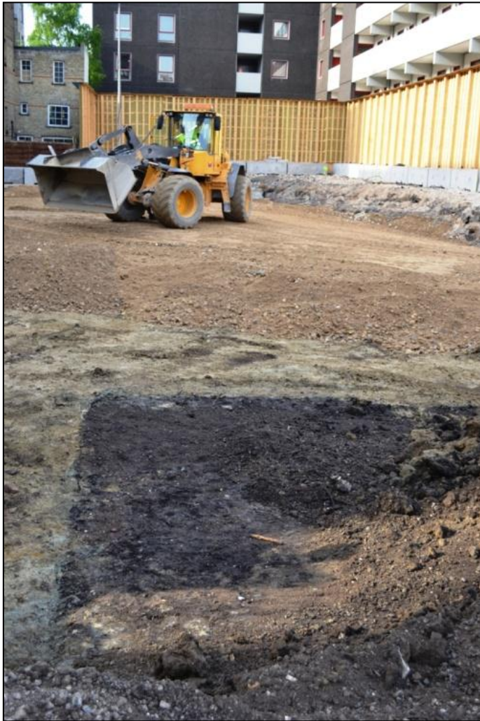
Figure 20. The dark rectangular shape in the foreground marks the SE corner of the cut for the concrete bunker (1063). A fill of sterile sand was found below the thin layer of dark, re-deposited topsoil. The machine in the background is seen laying out stabilizing gravel on the exposed natural subsoil.
