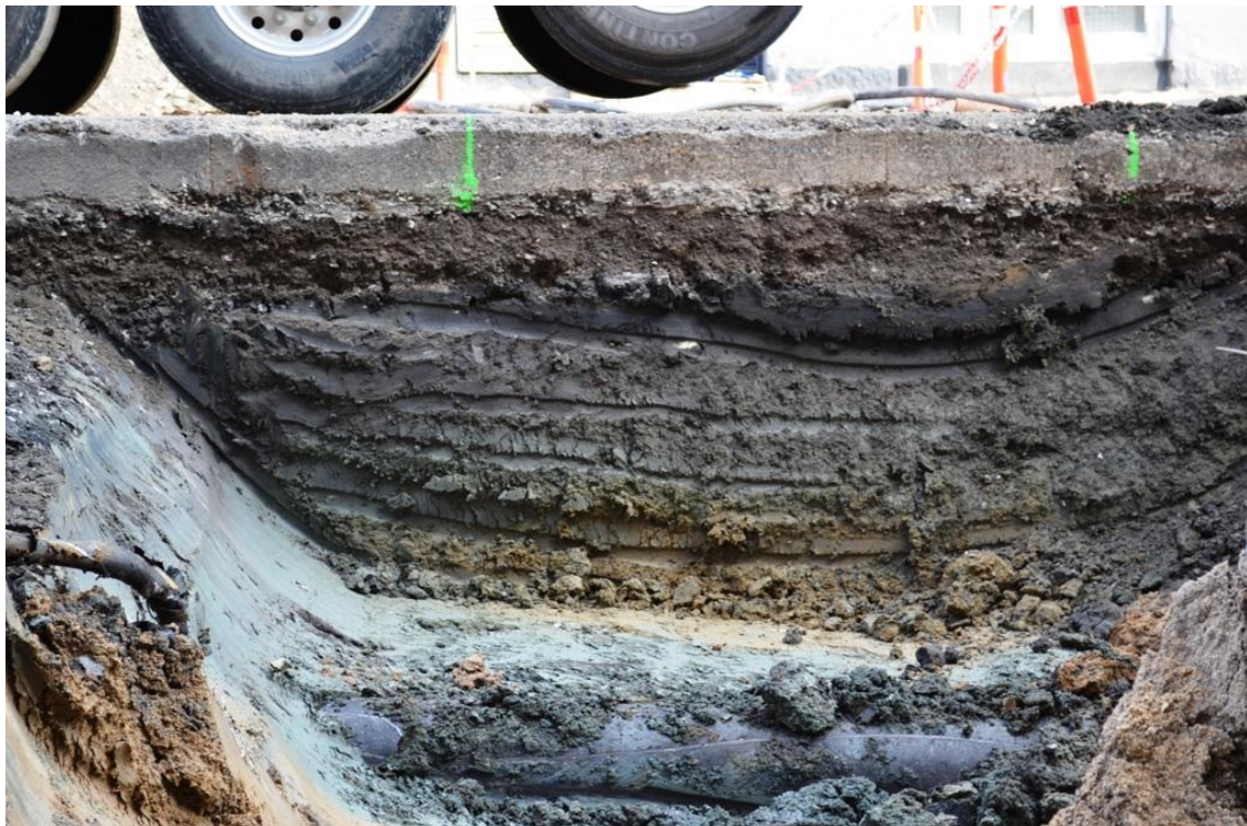
Figure 9. Machine-cut section parallel to Haraldsgade. The natural (yellow) subsoil is visible at the bottom of the section. One of the many pipes can be seen in the foreground.
