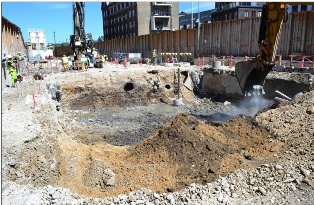
Figure 6. Excavation of the service shaft in progress seen towards the northeast. At the bottom of the trench is the grey sand of the former salt marsh and above it the dark brown leveling layers. Note the large gas pipe and other disturbances in the middle and to the right in the trench.
