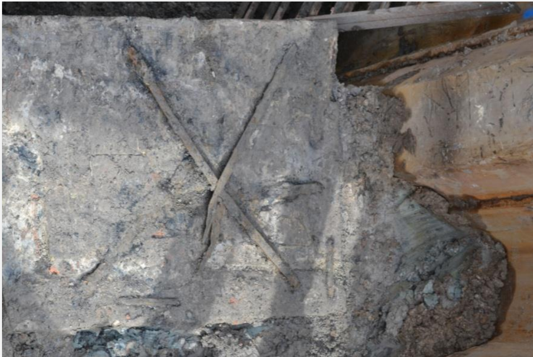
Figure 25. The picture shows one of the iron crosses and the iron clamps that holds together the bridge pillar (the picture is top – down). Københavns Museum, 2015.
