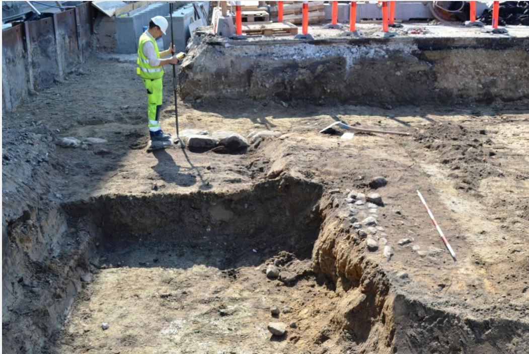
Figure 22. Work shot of the foundation and the paved surface to the right in the picture.
