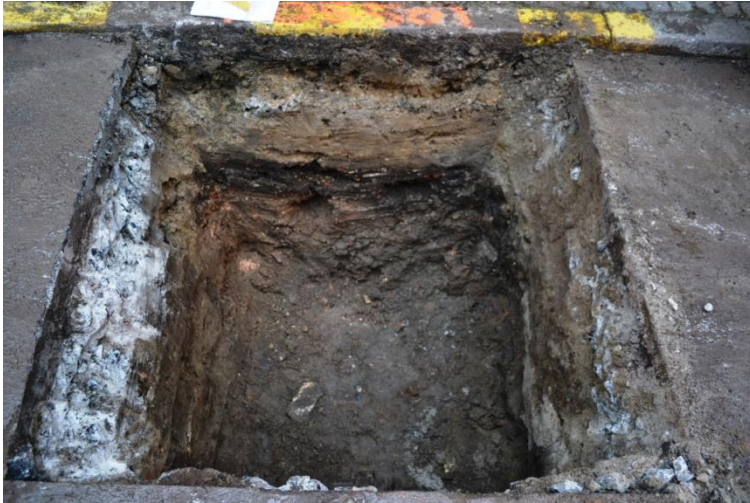
Figure 20. Trench Z100085. Dump layer SD100086 can clearly be seen as a dark horizon in the section.
