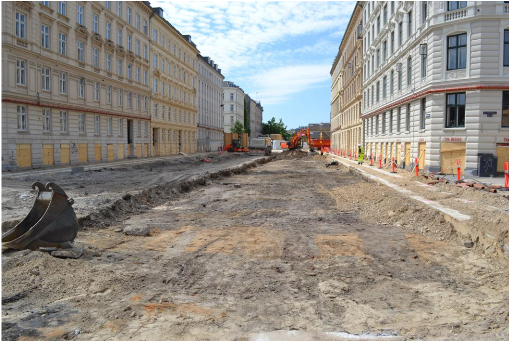
Figure 9. View towards west of the upper levelling layers S6 within the Guide wall trench.
