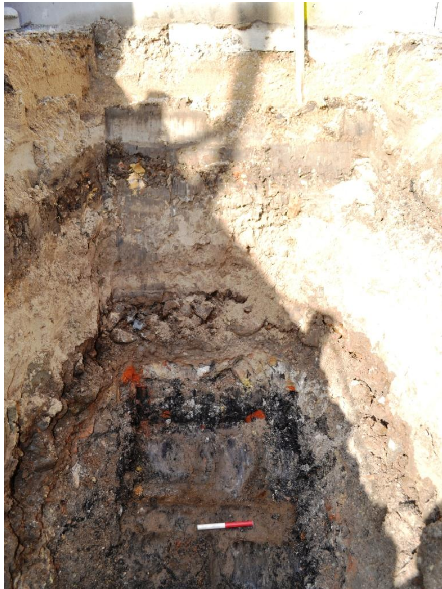
Figure 11. Section in pit for crane foundation at Reventlowsgade showing the cobble stone layer (blue arrow) and the sett paving with the drainage gully (yellow arrow).
